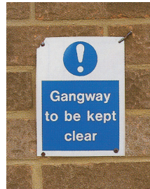
Safety sign has broken, splitting corners.
